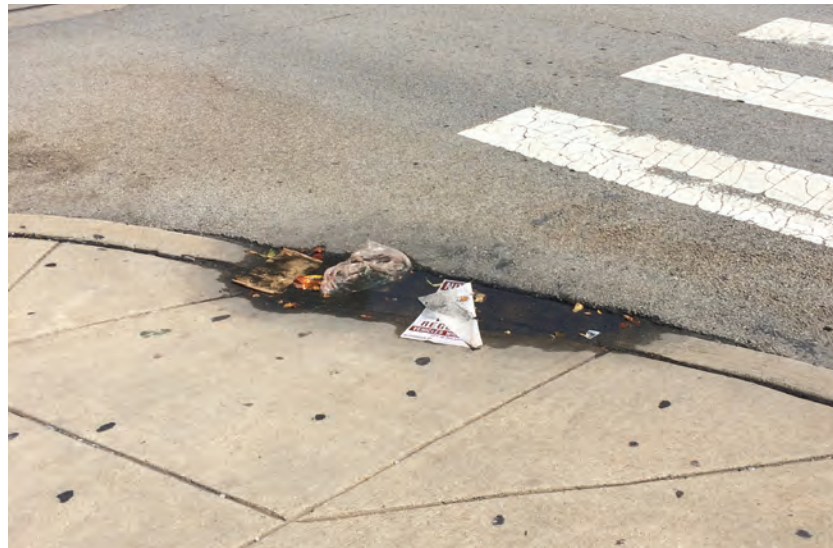
Below: Many of the curb ramps in the study area are not compliant, and several have drainage issues that make it difficult for pedestrians to cross. Source: DVRPC, 2017
