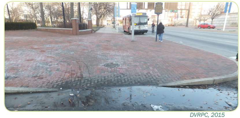
FIGURE 14: Non-ADA-compliant curb ramps and stormwater drainage issues
