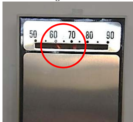
Figure 5: Malfunctioning Manual Baseboard Thermostat
