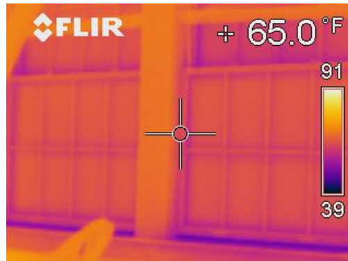
Figure 7: Second-Floor Office Windows, with insufficient closure and cold air infiltration
