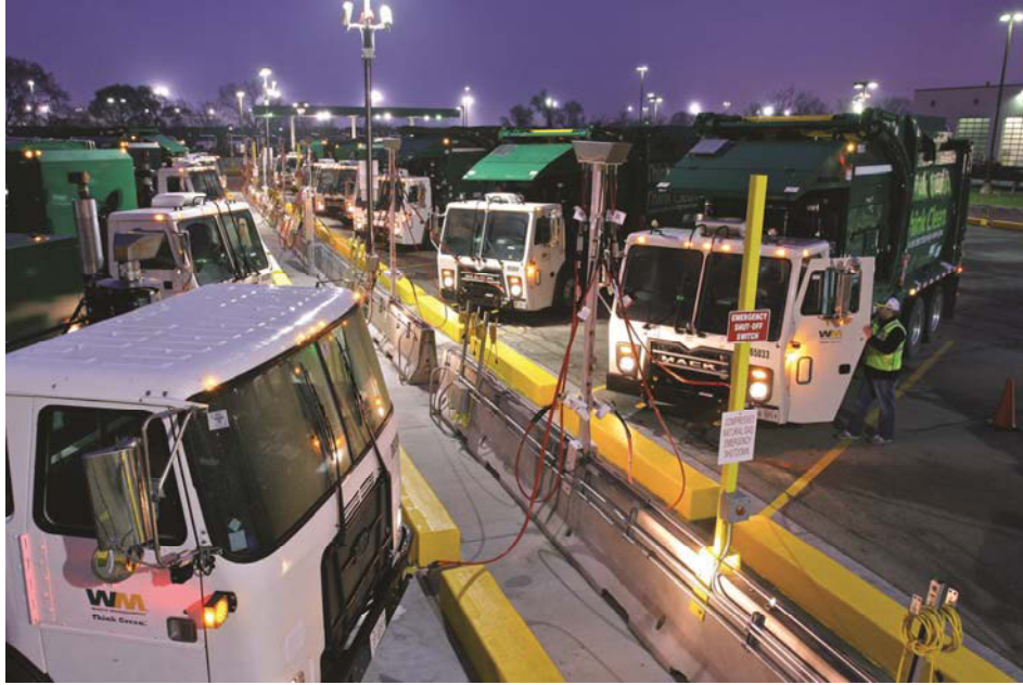
Figure 22. Waste Management time-fill compressed natural gas station in Chicago
