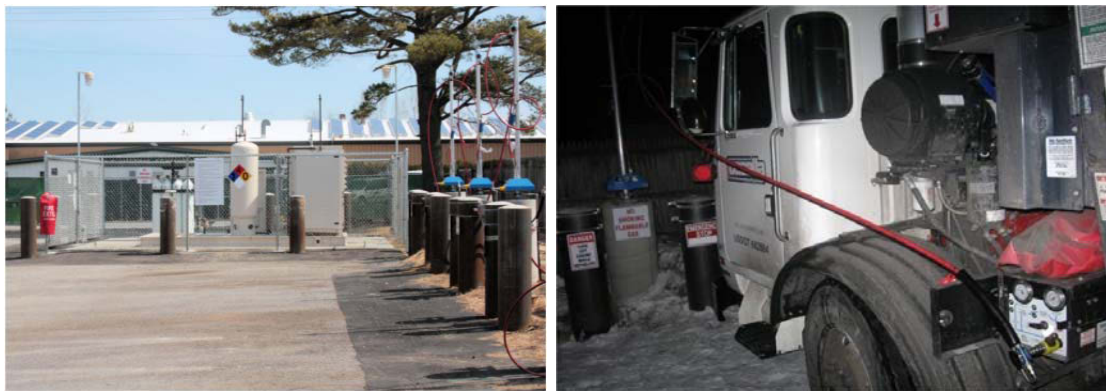
Figure 20. Casella Waste Systems time-fill compressed natural gas station for refuse vehicles
