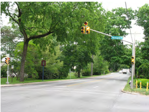
Consider upgrading these traffic signal heads at Remington Road.
