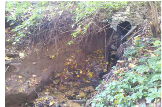
Erosion at Grange Field and County Open Space.
