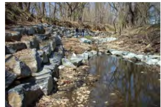
Rock pack and flush cut stream restoration. Photo: Montgomery County, Maryland DEP
