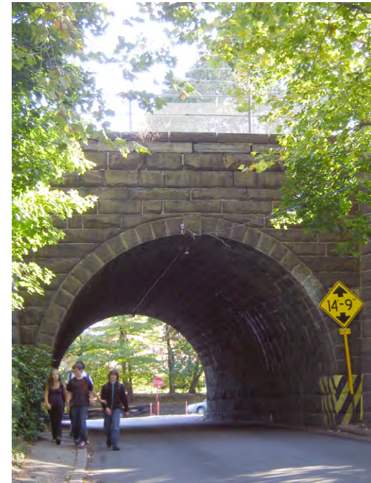
The historic rail tunnel is not pedestrian-friendly due to the narrow sidewalk.
