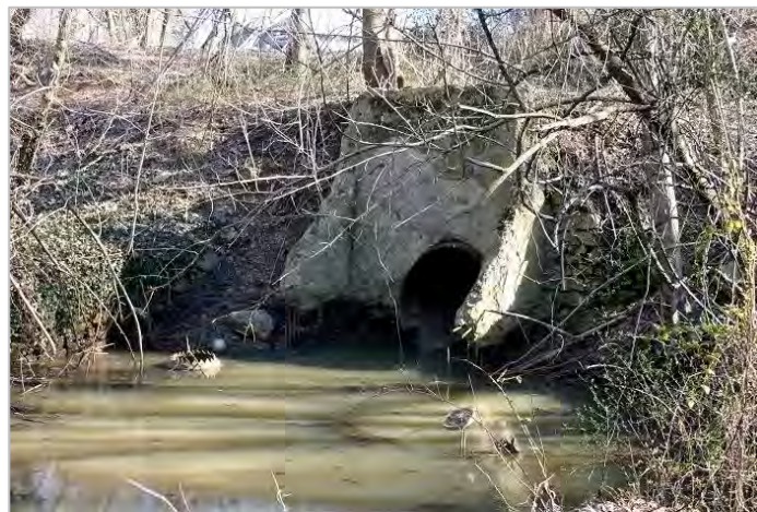
An Impaired Stormwater Outfall on Church Run
