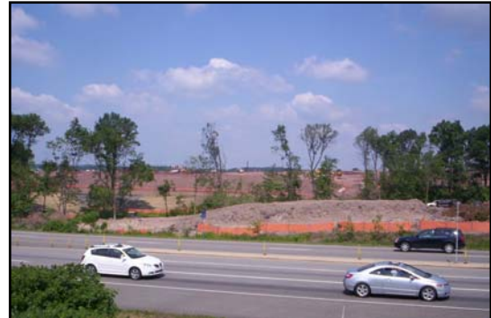
Pictured: Construction of the new Upland Square retail development begins in West Pottsgrove Township.
