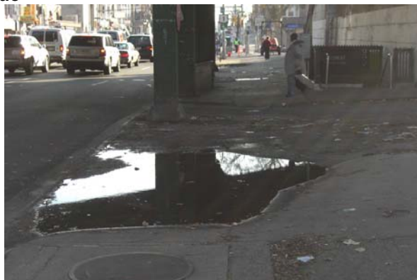
Unsafe pedestrian environment beneath underpass at Fishers Lane (See locations 9 and 10)
