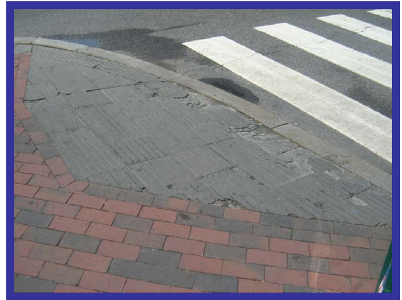
Damaged curb ramp common at many intersections in the corridor
