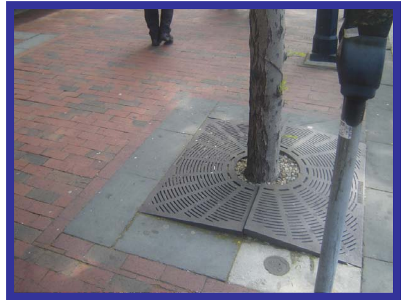
Tree grate lifting
