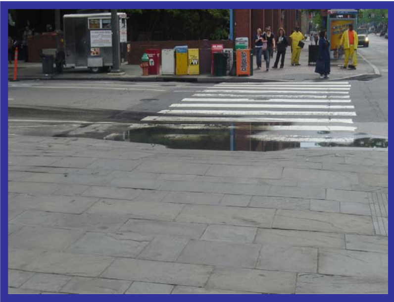
Pooling at the northwest corner of the 5 th Street intersection
