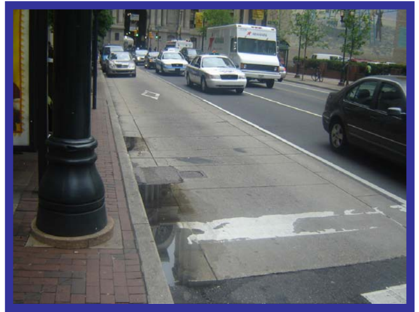
Pooling at the bus stop near the 13 th Street intersection
