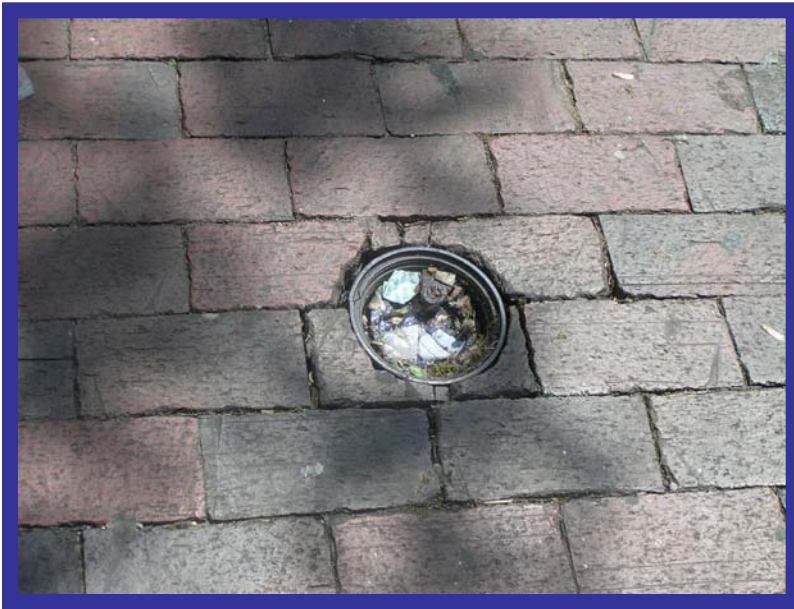
Cover removed from utility shut-off access
