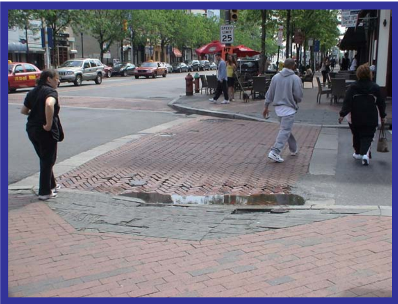
Pooling at the southwest corner of the 3 th Street intersection
