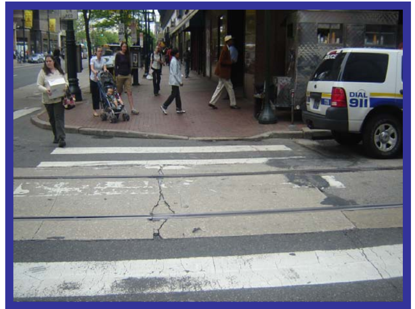
Deteriorating pavement across 12 th Street
