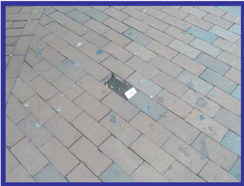
Missing brick on the sidewalk
