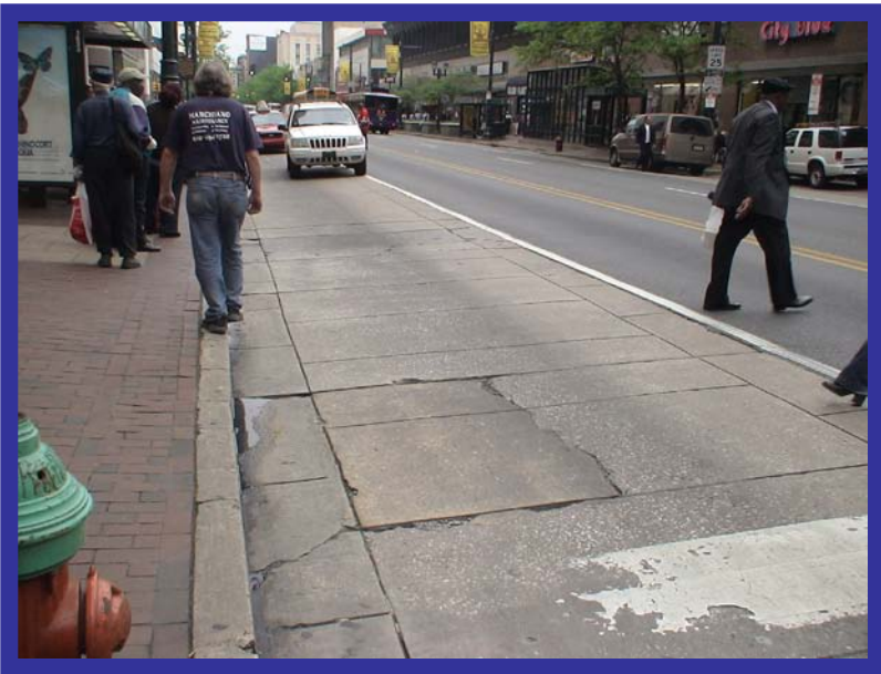
Deteriorating pavement between 13 th and Juniper Streets
