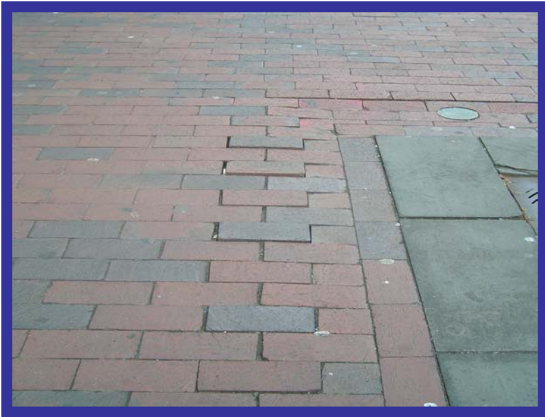
Loose bricks on the sidewalk
