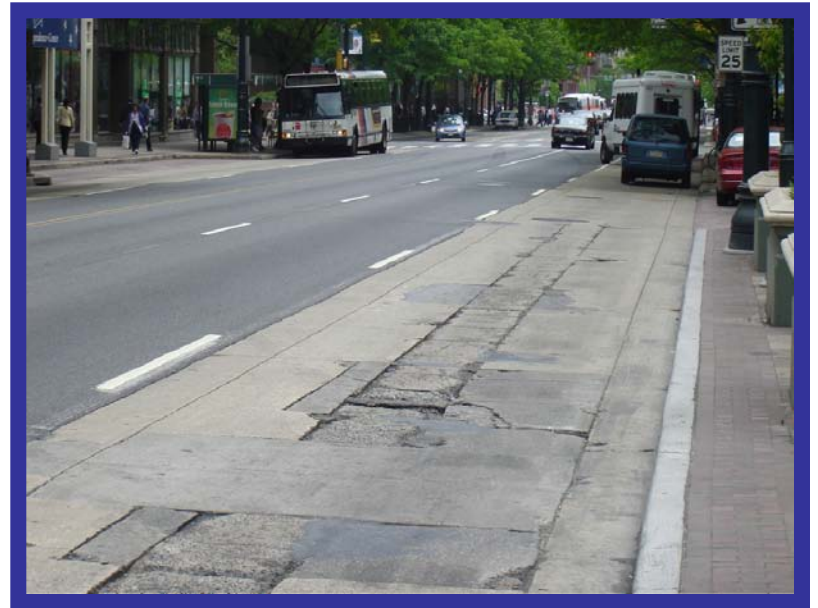
Deteriorating pavement between 7 th and 8 th Streets
