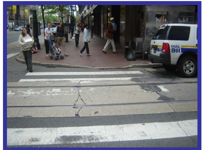
Faded crosswalk pavement marking and deteriorating pavement at 12 th Street
