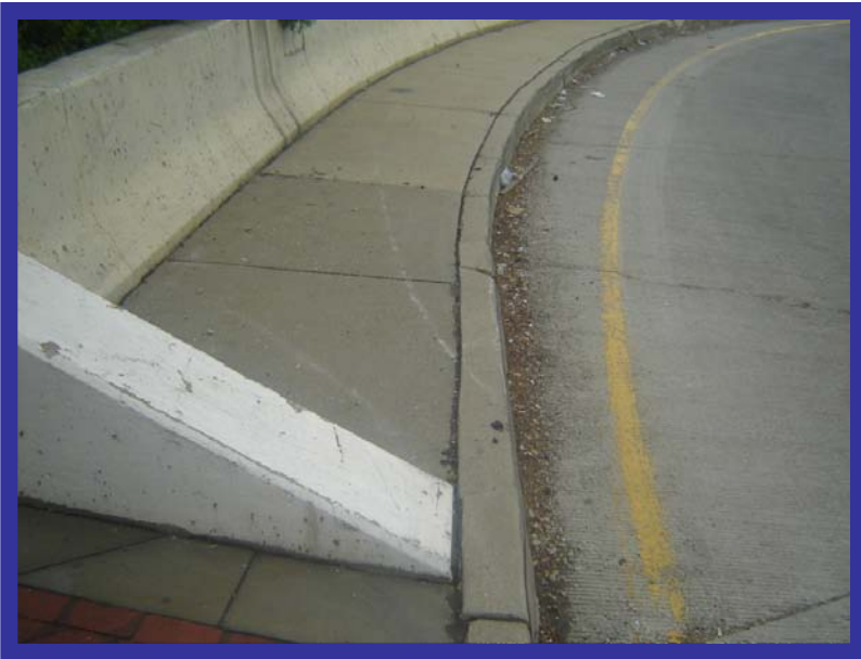
Damage to the walls of the I-95 southbound ramp
