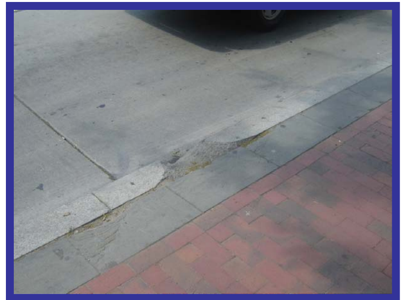
Damaged curb between 2 nd and 3 rd Streets
