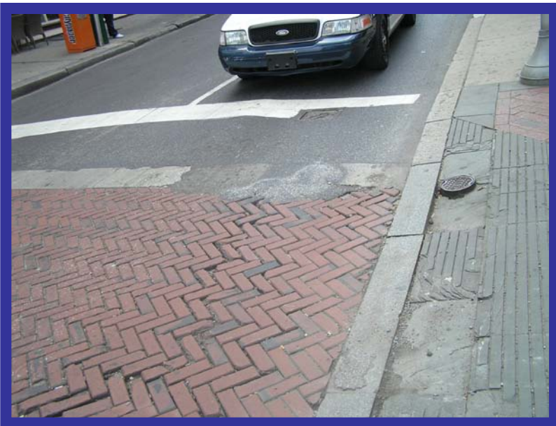
Damaged curb ramp common at many intersections in the corridor
