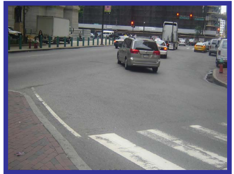
No pavement marking to guide motorist on Juniper Street, north of Market Street
