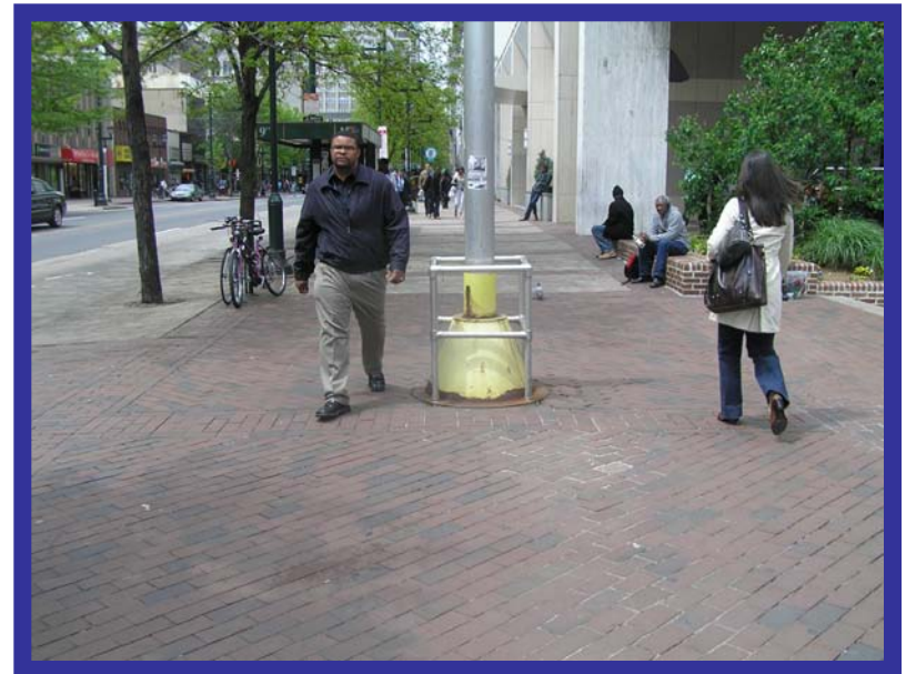
Vent in the middle of the sidewalk between 9 th and 10 th Streets
