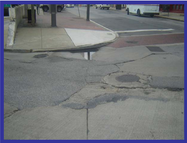
Deteriorating pavement at the entrance to I-95 southbound ramp
