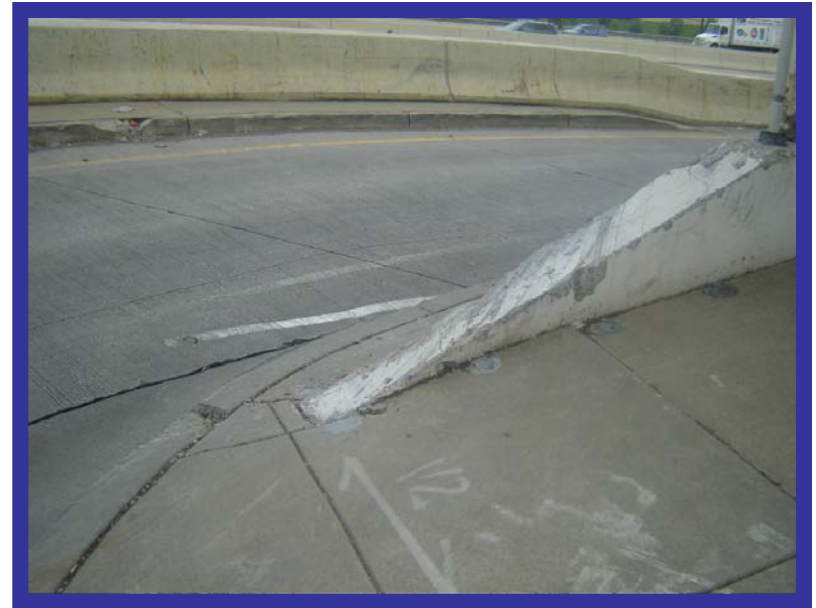
Damage to the walls of the I-95 southbound ramp
