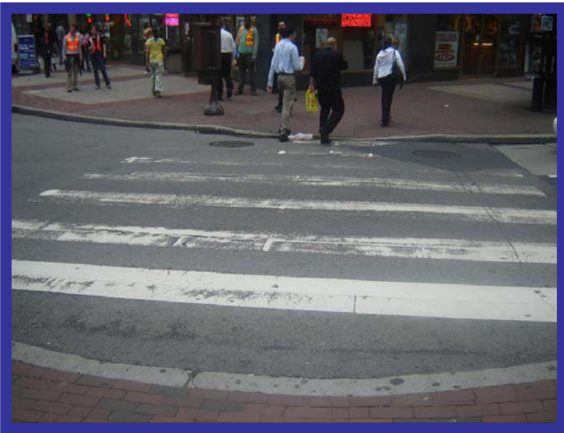
Faded crosswalk pavement marking at Juniper Street
