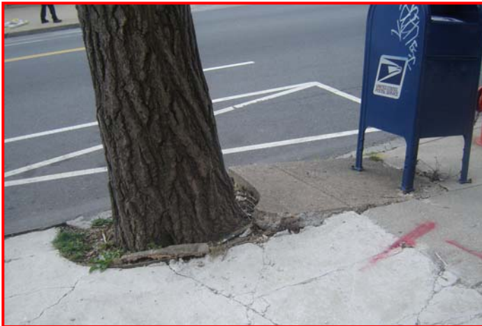
Tree roots dislodge sidewalk pavement
