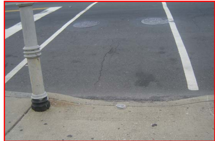
Curb ramp – not ADA compliant, uneven with roadway pavement
