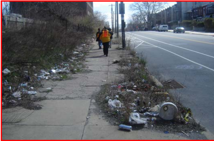
Trash and debris in sidewalk and drainage grates
