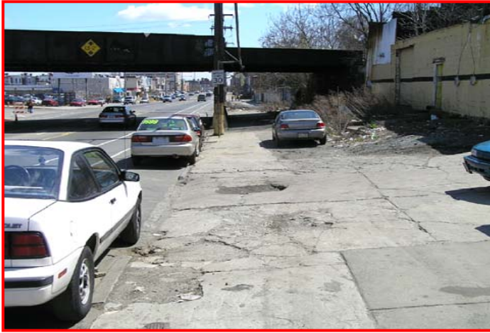
Sidewalks are cracked and rutted, vehicle parked on sidewalk
