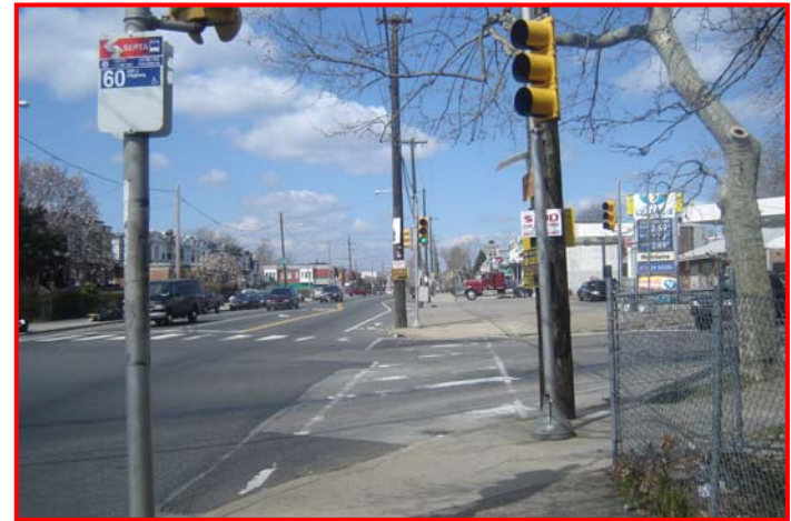
Faded crosswalk markings
