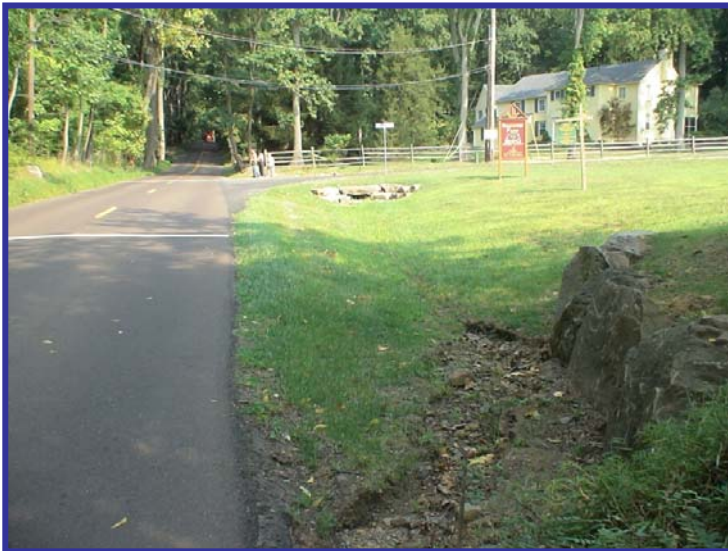
Edge of pavement drop off and drain at Rockwood Path
