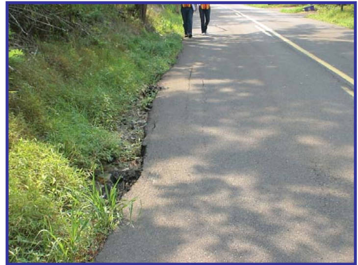
Edge of pavement drop off and deterioration on Aquetong Road west of Cover Bridge Road
