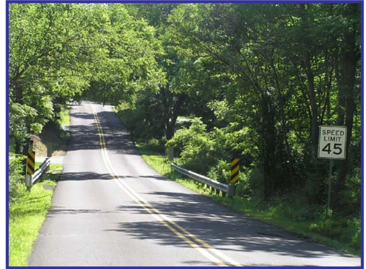
Narrow pavement of Aquetong Road west of Sugan Road, chevron signage at guide rail
