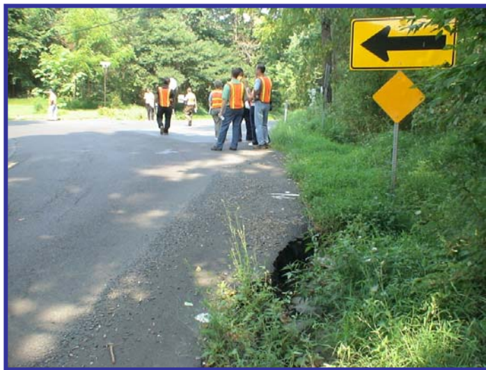
Edge of pavement drop off and deterioration on Aquetong Road east of Sugan Road
