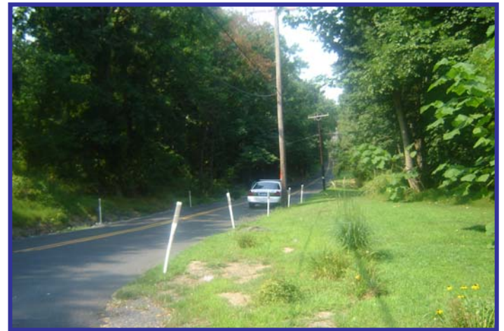
Leaning delineator pole on Aquetong Road west of Sugan Road
