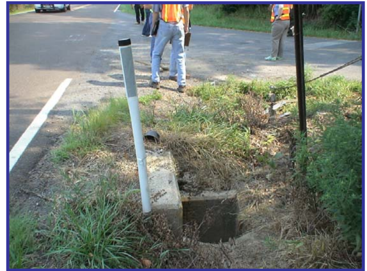
Inlet at the intersection of Old Windy Bush Road and Windy Bush Road
