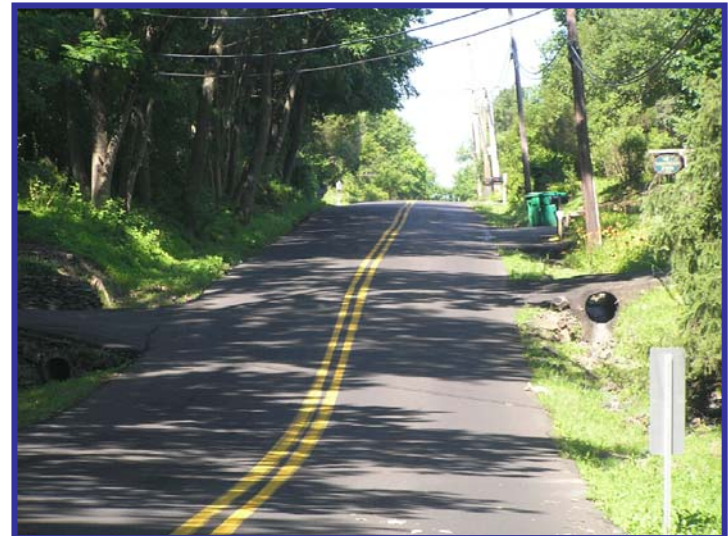
Oversized drain pipe at private property driveway on Aquetong Road west of Sugan Road
