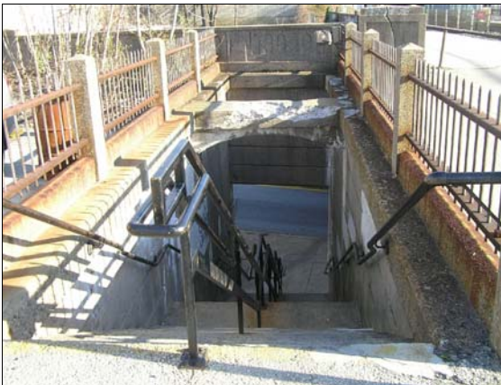
A stairwell on the north side of Glenside station leading to Easton Road. The sidewalk below has no guardrail, however, to protect pedestrians from traffic.
