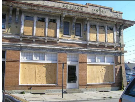
The fire-damaged Roberts Block building just north of the station could serve as an anchor for commercial redevelopment.
