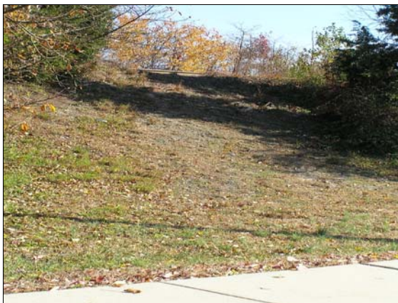
The lack of an underpass forces pedestrians to find other, more dangerous ways of crossing over the tracks. This worn path on the southern side of the tracks is evidence.
