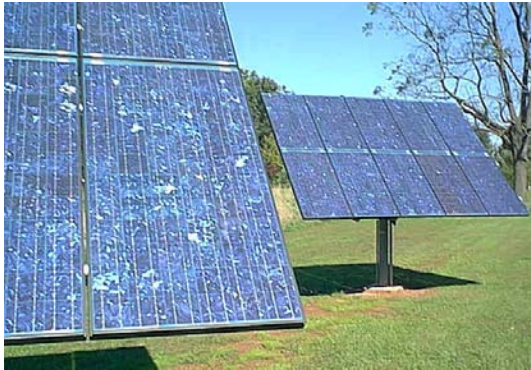
Photovoltaic Technology, Chester County
