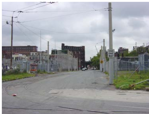
PECO substation along Noble Street
